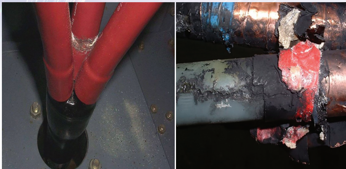
Partial Discharge Damage at Field Terminations as a Result of Poor Workmanship
